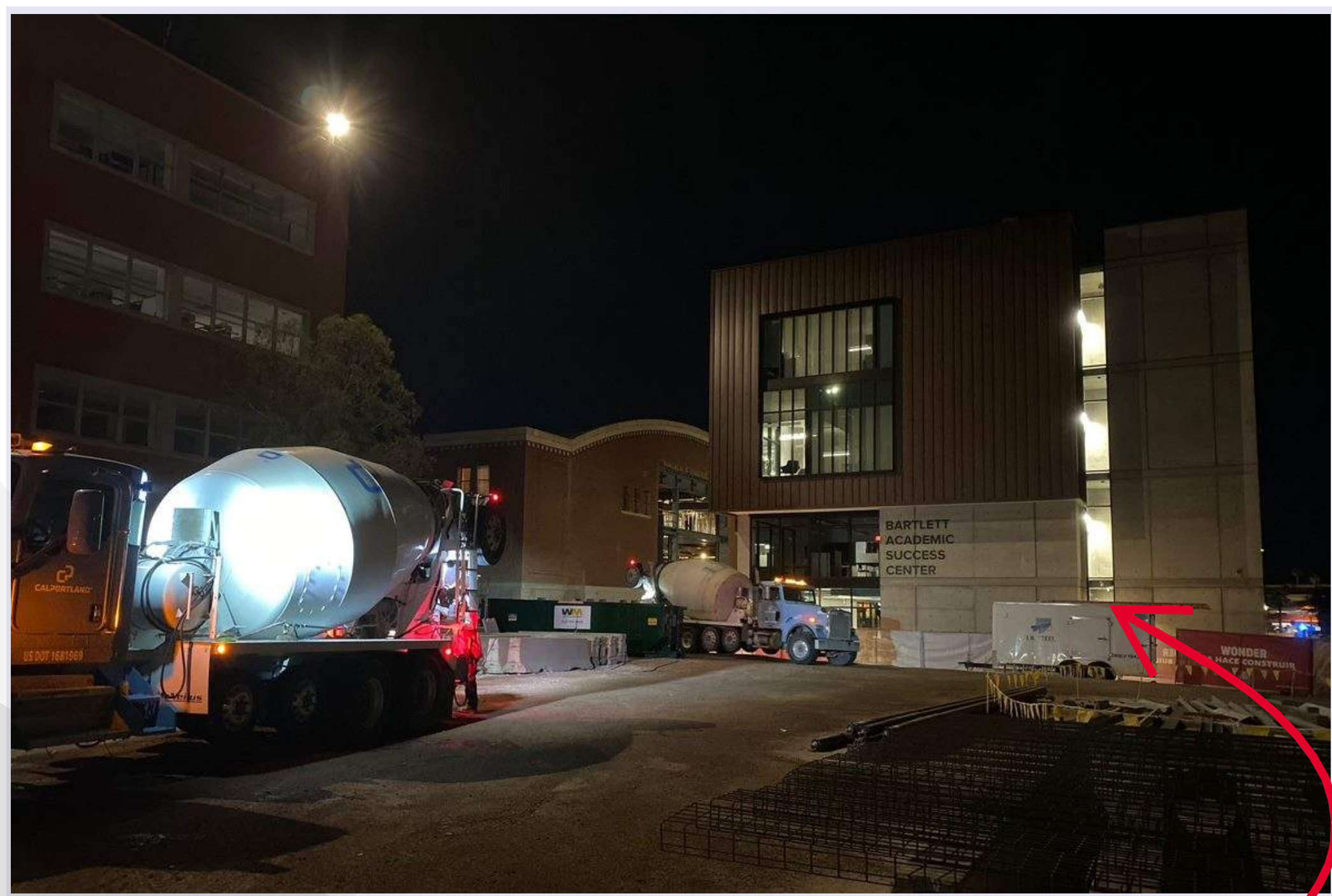
Concrete trucks for the level 1 slab on grade in the Bear Down Gym. FUN FACT: Concrete is typically placed at night in Arizona so hot temperatures do not interfere with the curing process. Night placements are also often required due to concrete availability for large quantity orders.
