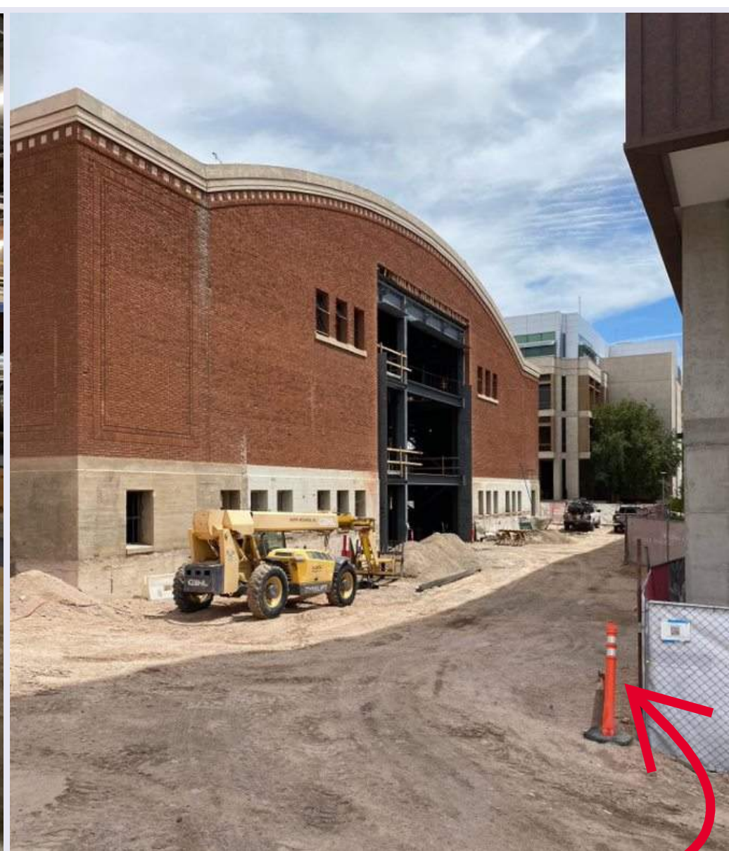
The diagonal building braces have been removed now that the structural steel and elevated concrete decks have been completed inside the building. Bridges will be added to connect Bear Down Gym to the new Bartlett building.
