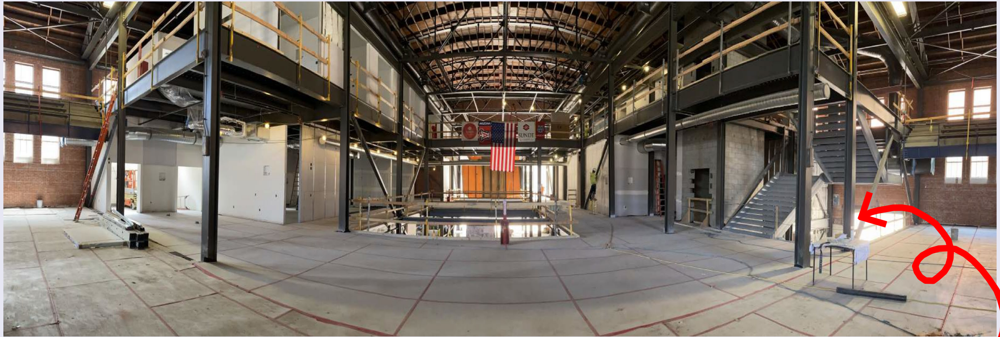
Inside the main entrance standing on the historic gym floor, looking south. Level 3 paint is underway, level 2 walls are receiving tape and texture, and the level 1 floor is being polished. The main stair is going in on the right.
