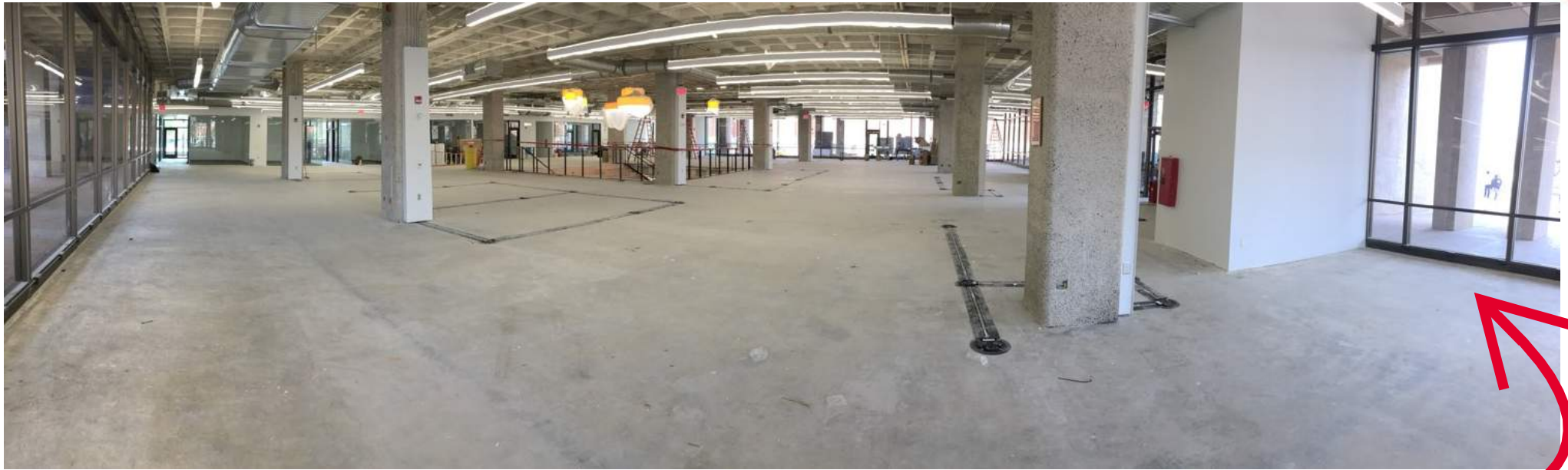
A PANORAMIC VIEW OF POD 'A' LEVEL 2 PROGRESS, FLOORING IS JUST ABOUT TO START!
