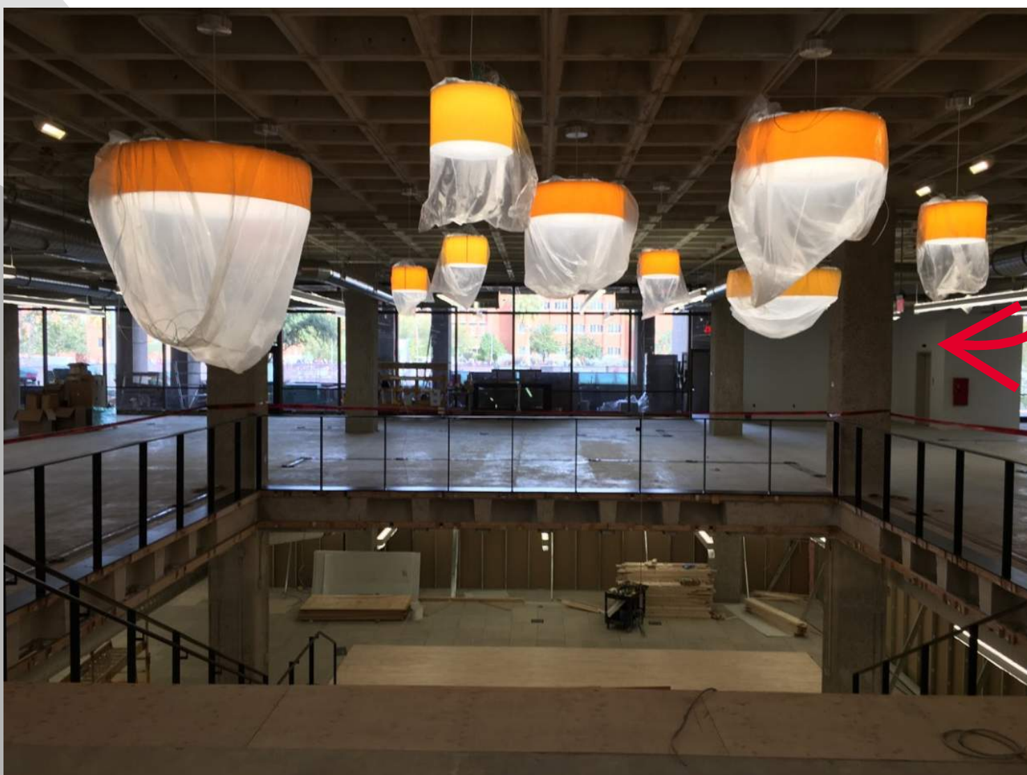
MONUMENT STAIR PROGRESS IS ONGOING WITH FLOORING AND GLASS IN THE RAILINGS!
