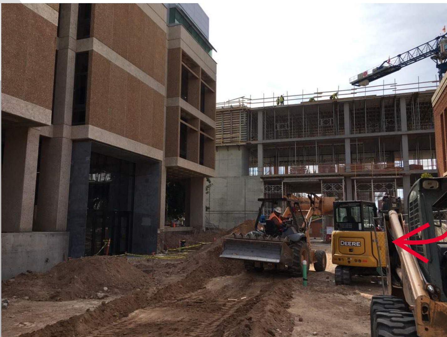
A VIEW OF THE GRADE PREPARATION OUTSIDE OF POD 'A', LOOKING SOUTH AT STUDENT SUCCESS BUILDING!
